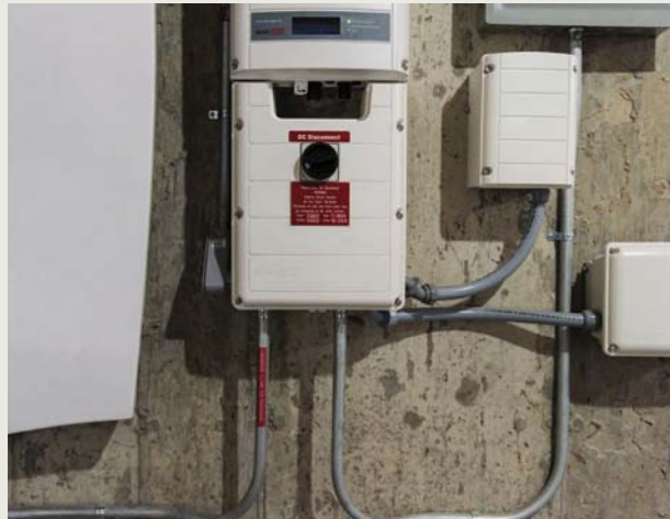
This wall battery system is installed in a residential garage. It stores electrical energy from a home solar electric system and can be used to power the home or an electric car.
