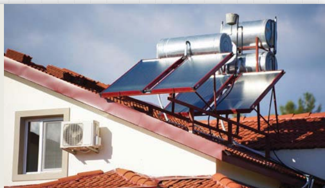
These solar water heaters convert electromagnetic energy into thermal energy.
